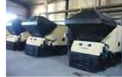
High-efficiency Heat only Boilers, Suuri-Keikaku, Mongolia
