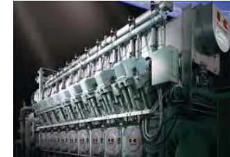
Co-generation system at factory, Toyota, Nippon Steel & Sumikin Engineering, Indonesia, Thai
