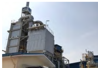
Waste to Energy Plant, JFE engineering, Myanmar
