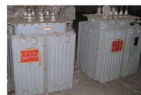
▲Devices containing PCB
