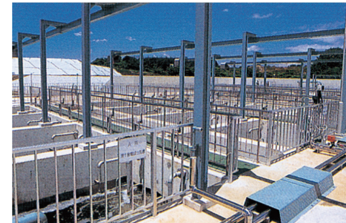
Wastewater treatment facility (contact aeration tank)
